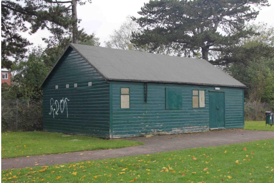
Poor quality changing facilities at Merstham Recreation Ground
