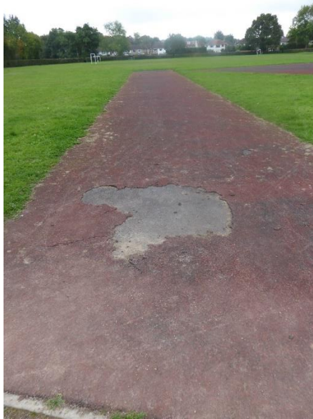
Battlebridge Athletics Track showing delaminated surface on the javelin run-up
